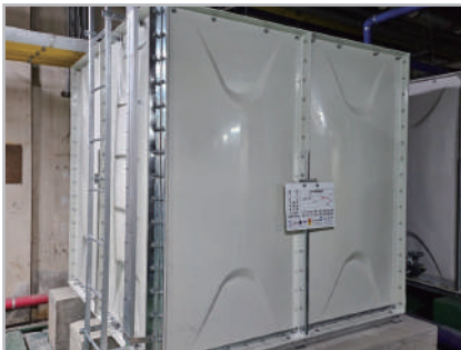
Finish, Tank Check
